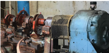
Above: Piston-pumping system to be replaced
