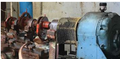
Above: Piston-pumping system to be replaced
